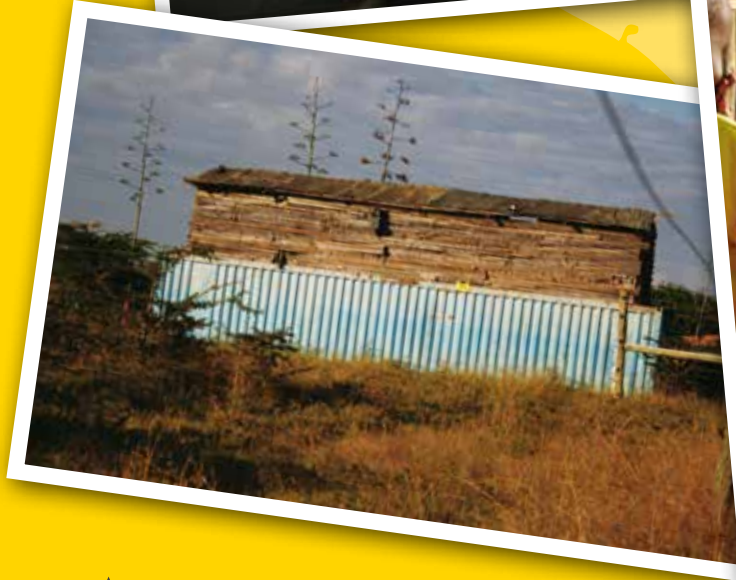
▲ It may not look like much but this local clinic, just down the road from the school, provides vital medical support and education for the local community, particularly in tackling HIV.
